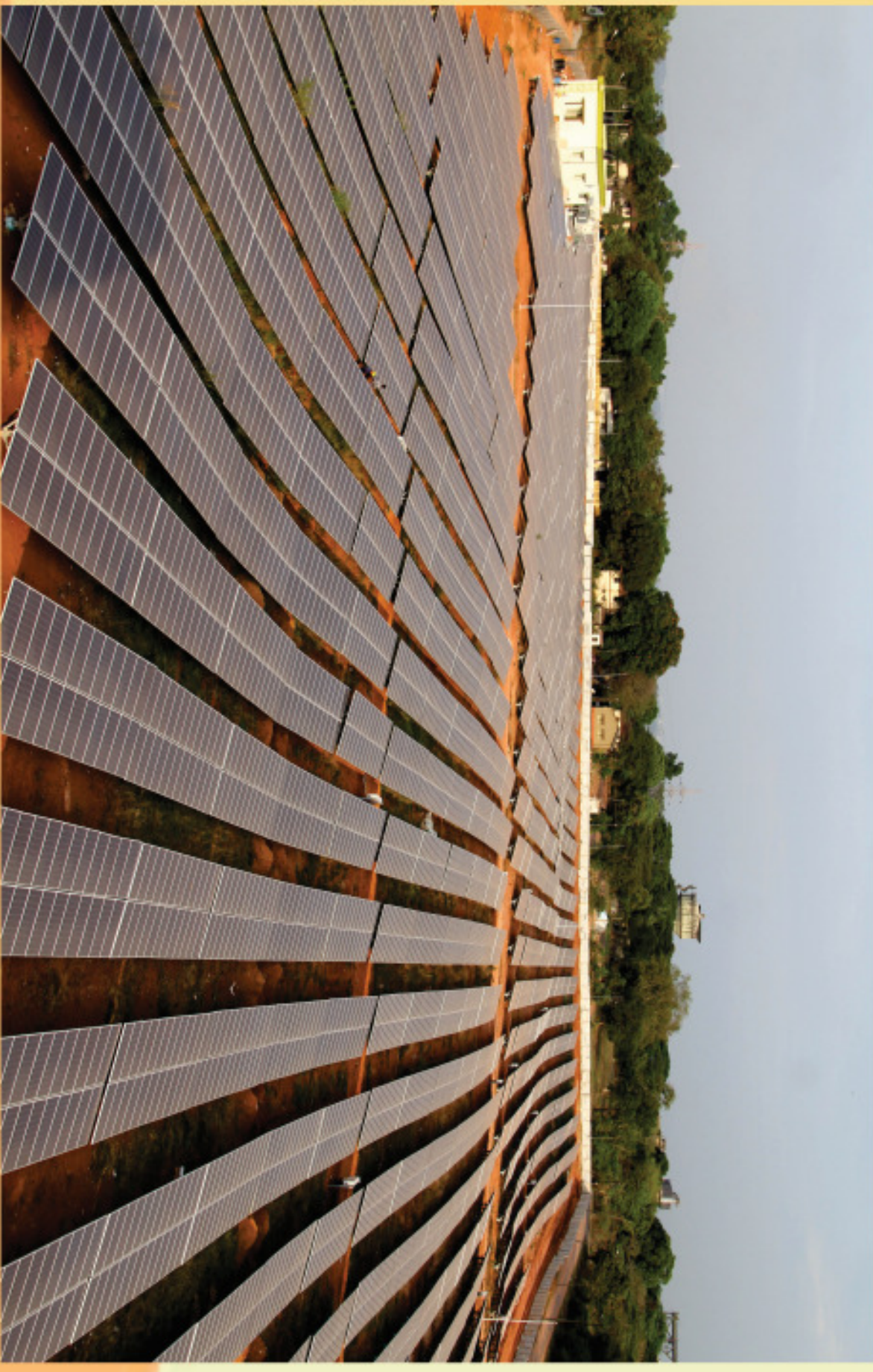
4 MW Solar Power Plant inside the Port Colony
